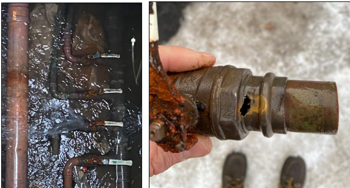
Water Leak Investigation (Feb. 20, Homestead Dr.)
