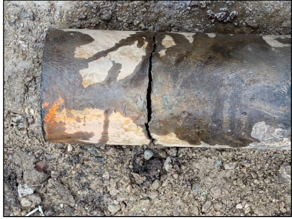
Break in the 6" water main
