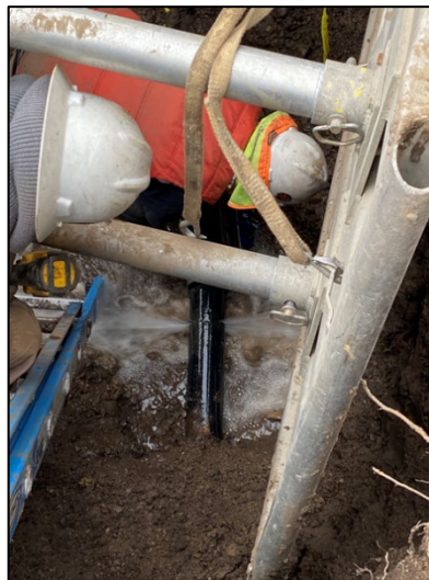
Water Main Leak (West Gore Creek Dr)
