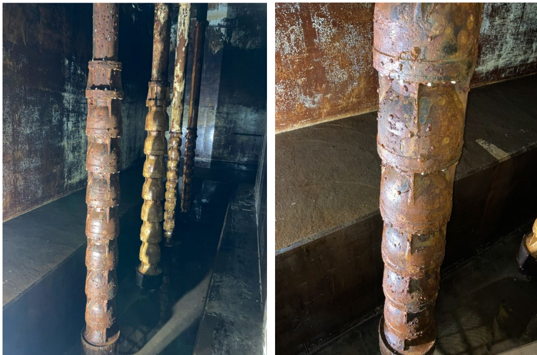
Finished water pump corrosion identified during routine wetwell inspection
