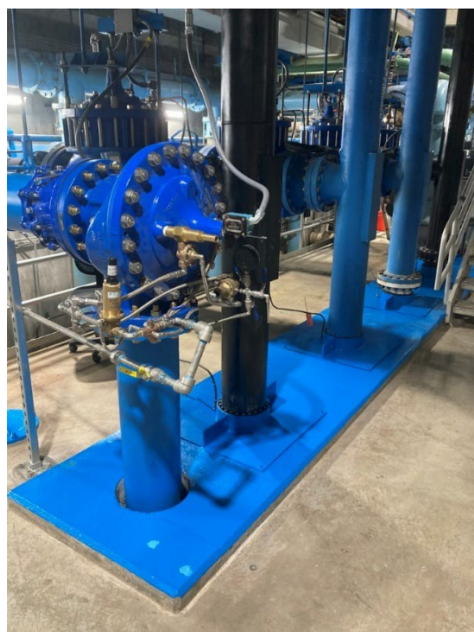
Surge anticipator valve in ADWF pump gallery
