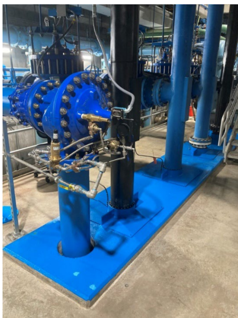
Surge anticipator valve in ADWF pump gallery
