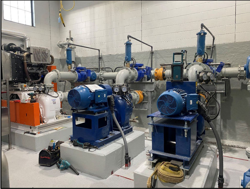
Pumps and piping in new lift station
