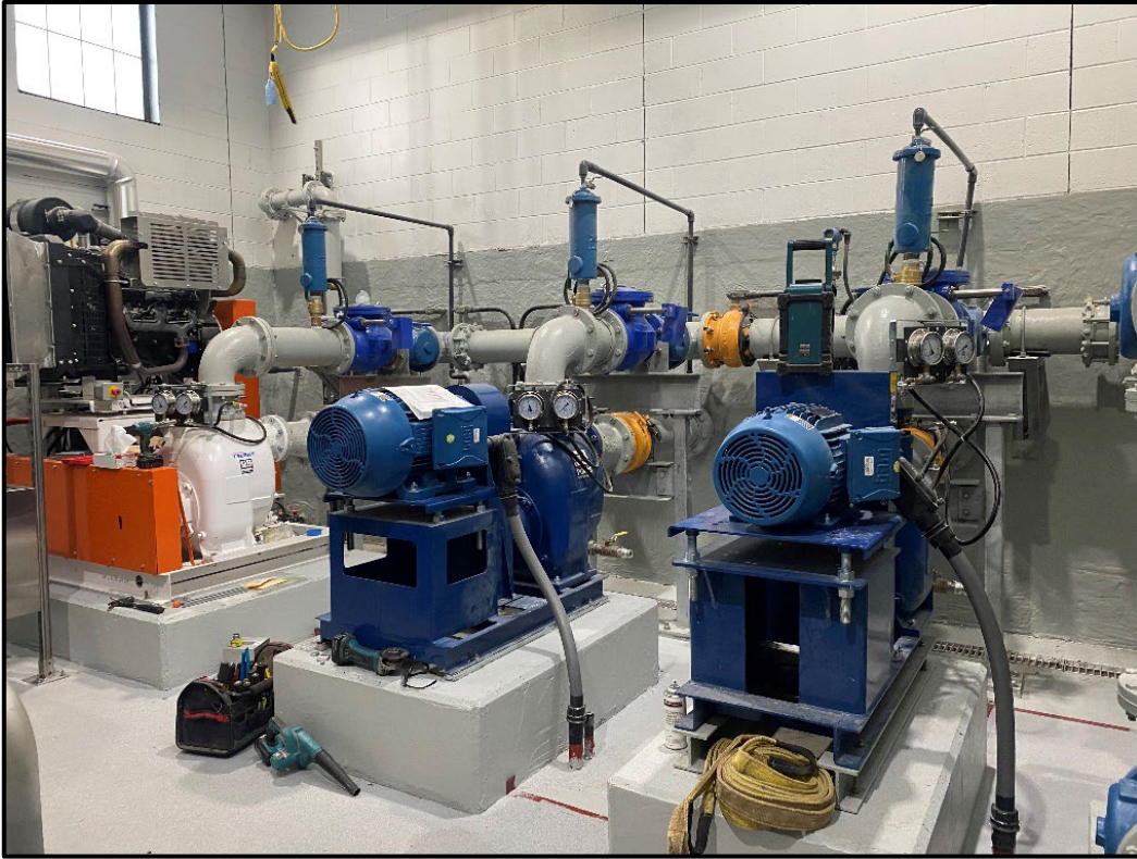
Pumps and piping in new lift station
