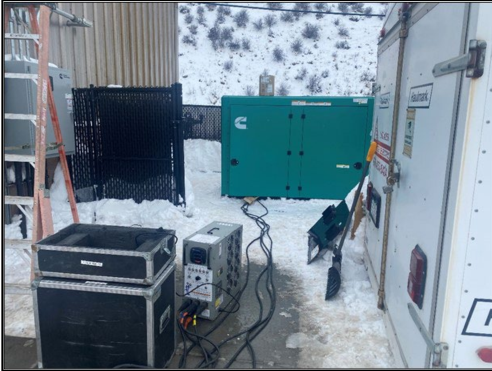
Load testing the new natural gas generator
