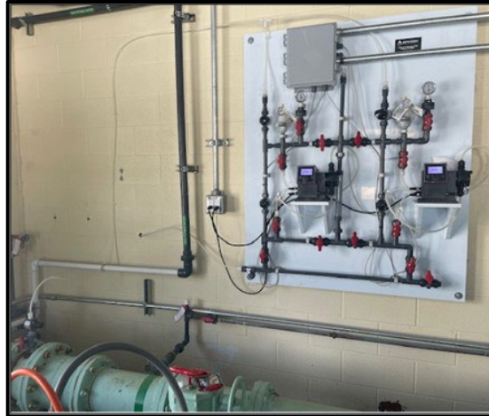
New backup chlorination feed panel at Berry Creek Wellhouse
