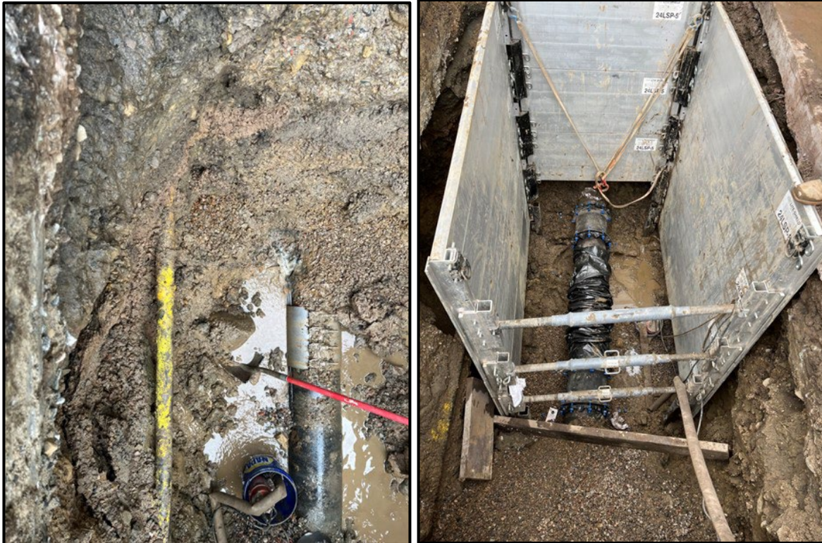
Beaver Creek water main repair (damaged pipe and failed repair clamp on left; pipe repair on right)
