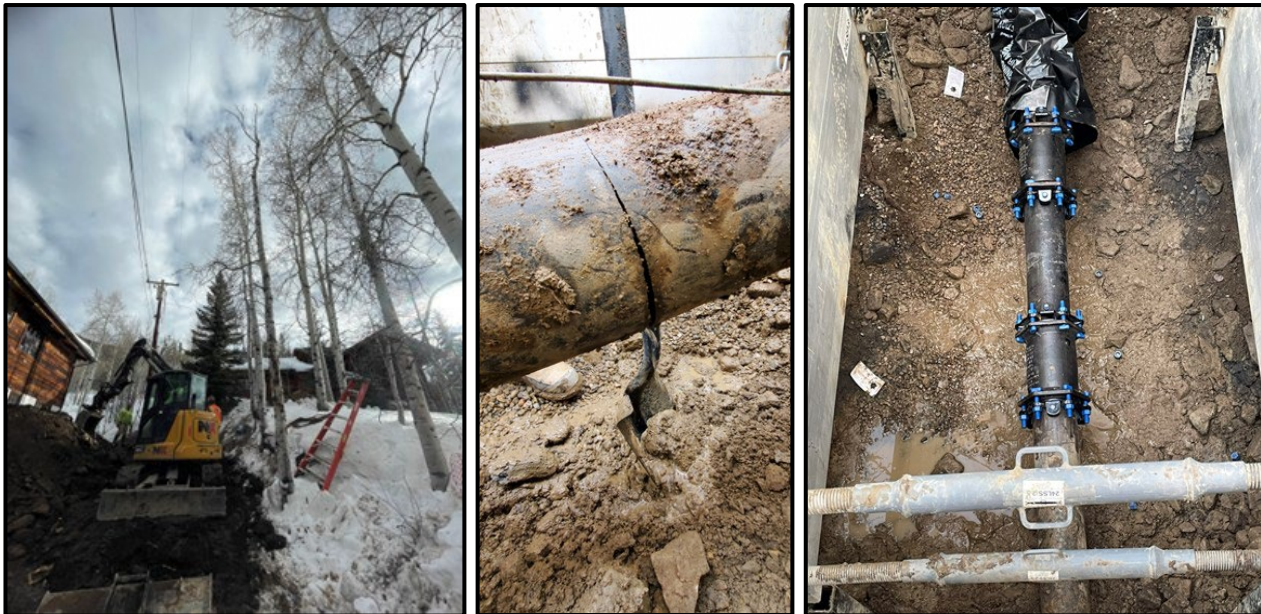
Matterhorn Circle water main repair (excavation left; pipe damage center, repair right)
