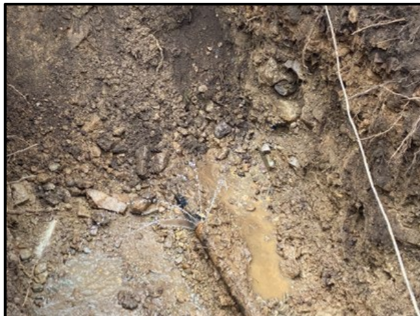
Damaged pipe and leak location
