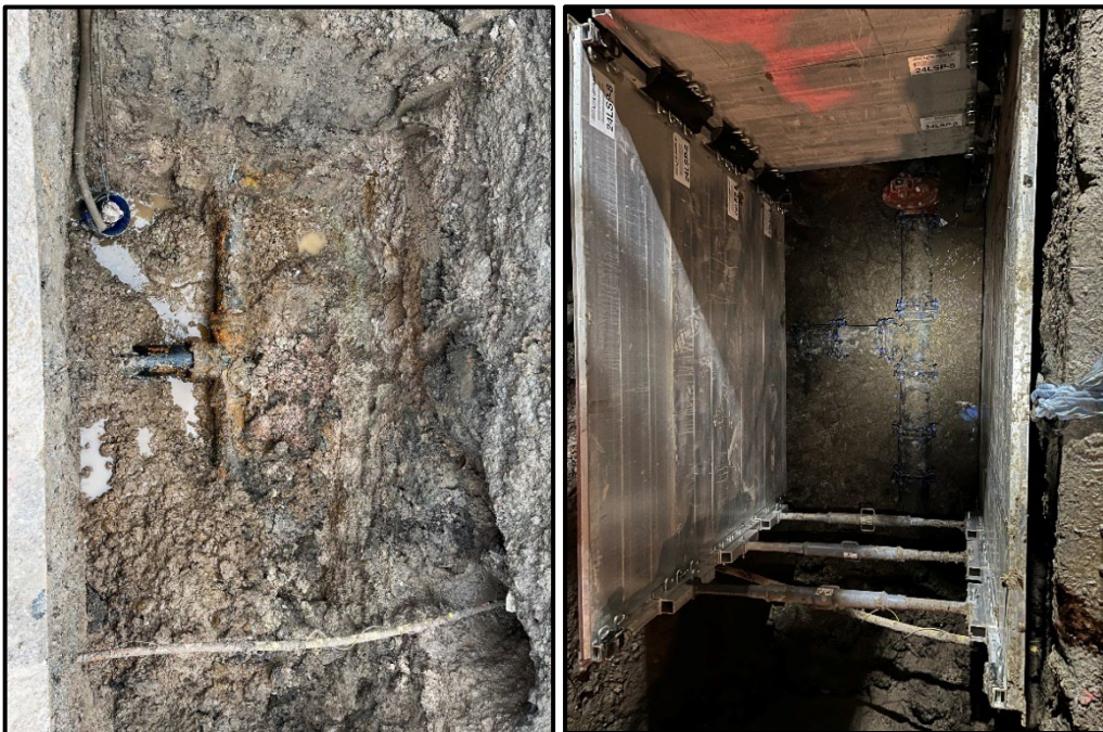
Wildridge water main repair (damaged pipe on left; new pipe and isolation valve on right)
