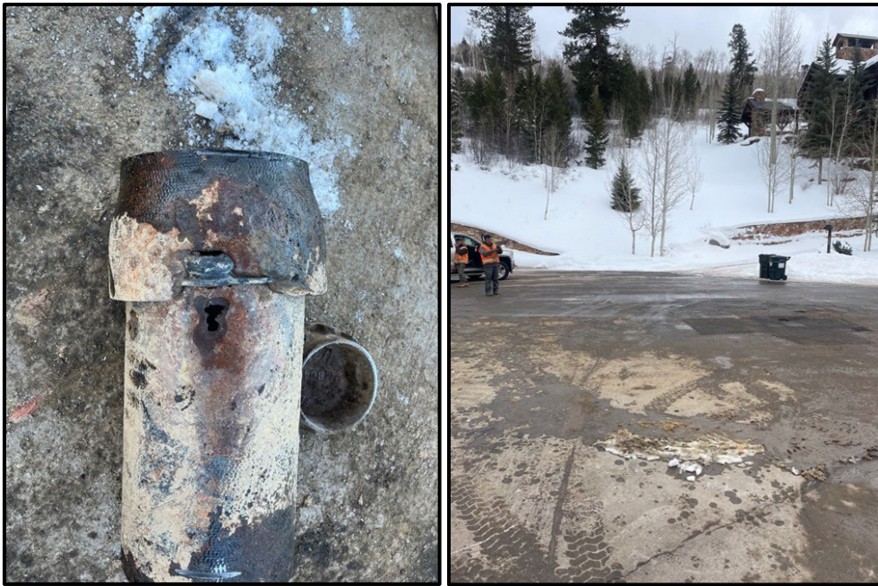
Arrowhead water main repair (damaged pipe on left; restored site on right)
