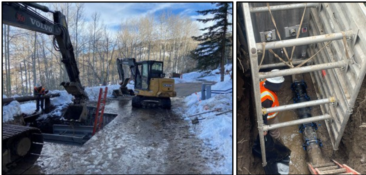
Bachelor Gulch water main repair (excavation on left; pipe repair on right)
