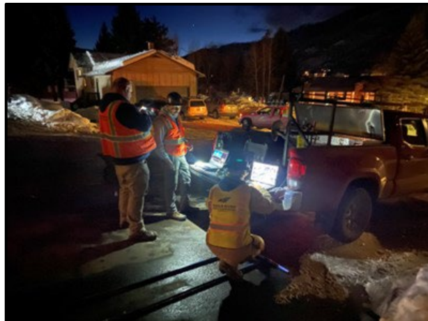
Field crew correlating leak location
