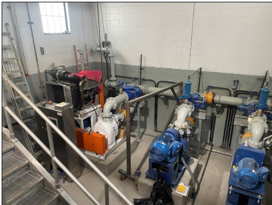
Engine-driven pump installation (shown on far left)
