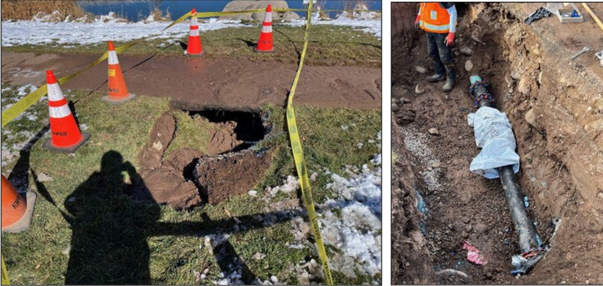
Berry Creek Well #2 raw water pipe repair (Oct. 30 – Nov. 1) Sinkhole damage near the pedestrian path (left); completed repair (right)
