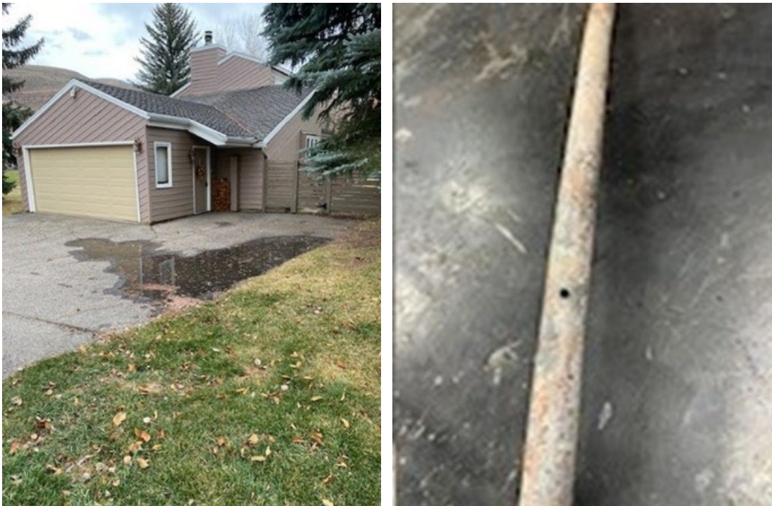
Water service line repair in Eagle Vail (Nov. 19-20) Water surfacing in driveway (left); hole in copper service pipe (right)
