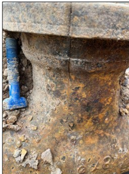
Cracked ductile iron fitting
