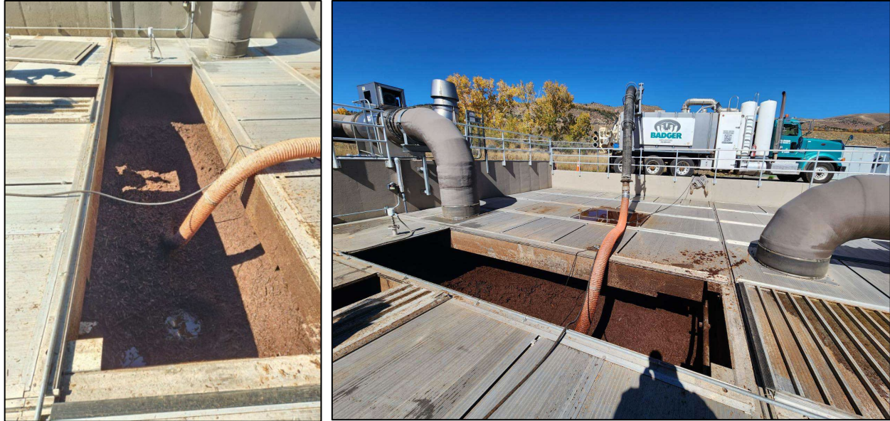
Media removal from EWW odor control biofilter
