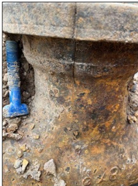
Cracked ductile iron fitting
