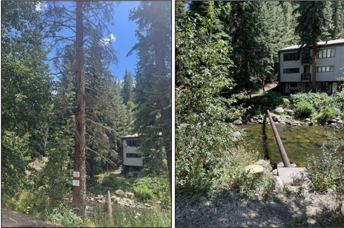
Tree removal to prevent damage to sewer collection main (before and after)
