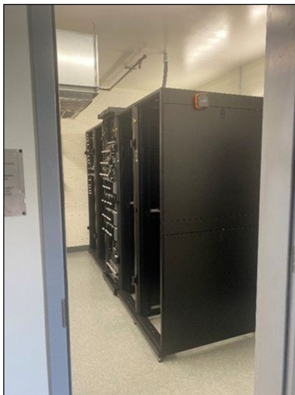
Server Commissioning at ADWF
