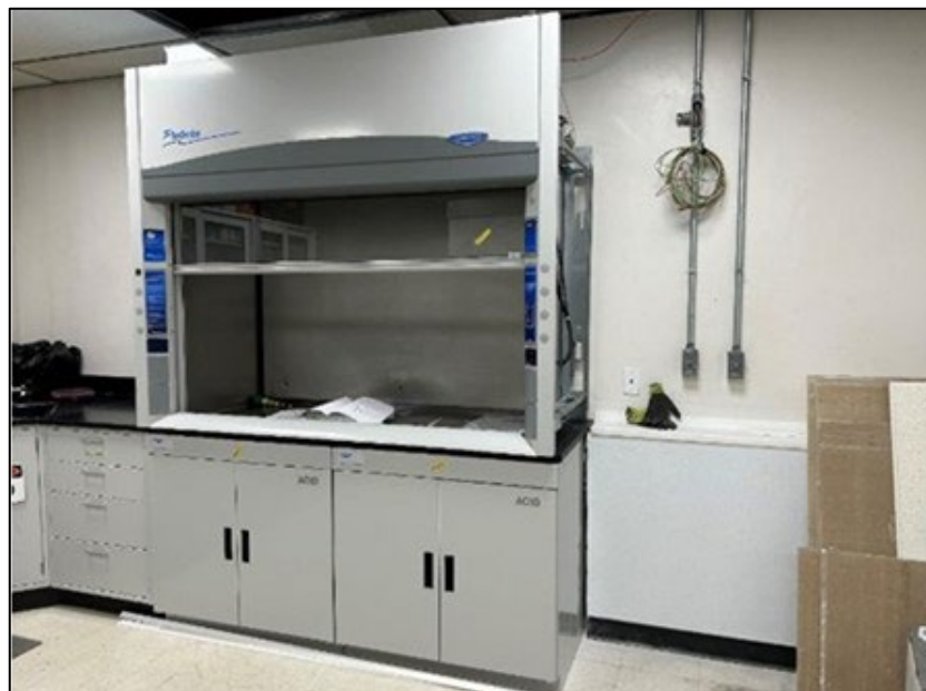
New Fume Hood
