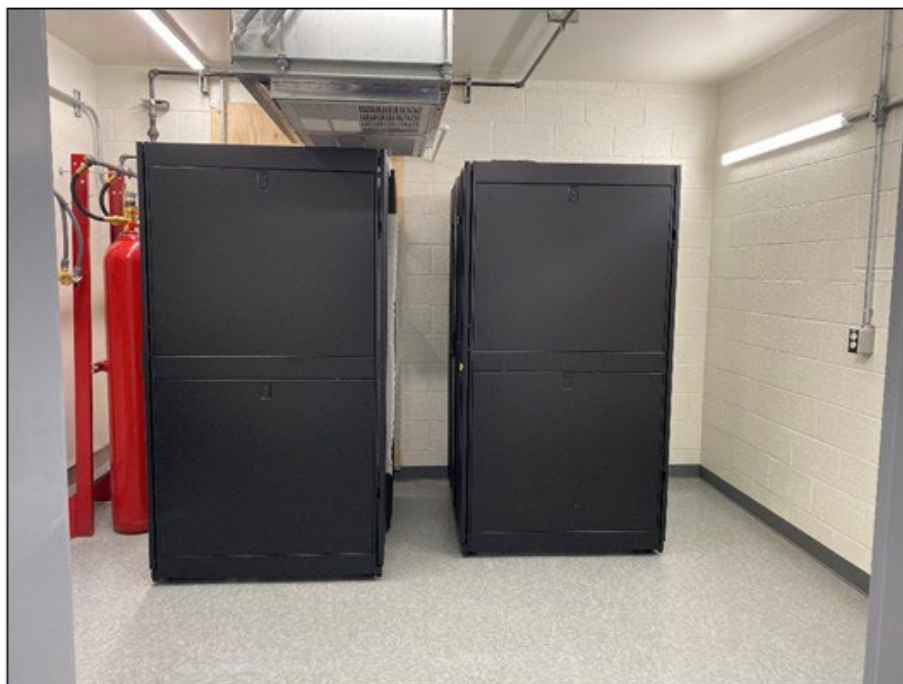
New IT server racks at ADWF
