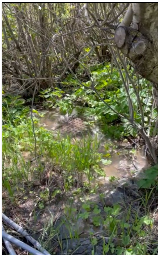
Surcharging Manhole (Jun. 10)
