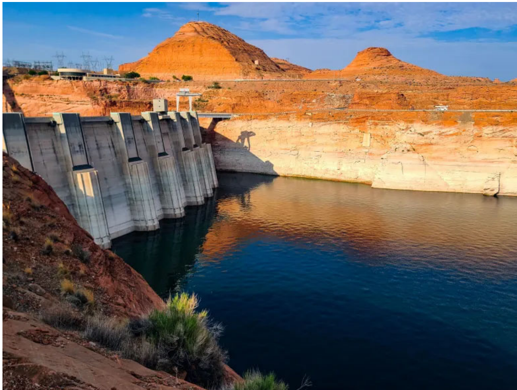
Glen Canyon Dam at Page, Arizona, holds back the massive Lake Powell. Since this photo was taken on Aug. 21, 2021, drought conditions in the West have led levels of water in the lake to drop near where the dam will no longer be able to generate electricity. (Bureau of Land Management)
