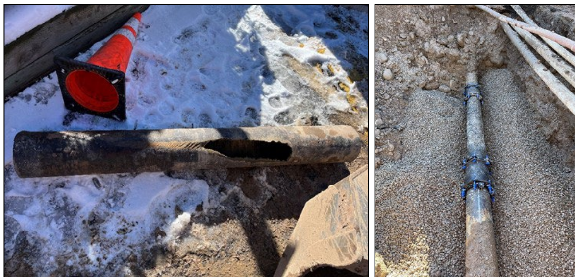
West Beaver Creek Blvd. water main repair (damaged pipe left, completed repair right)
