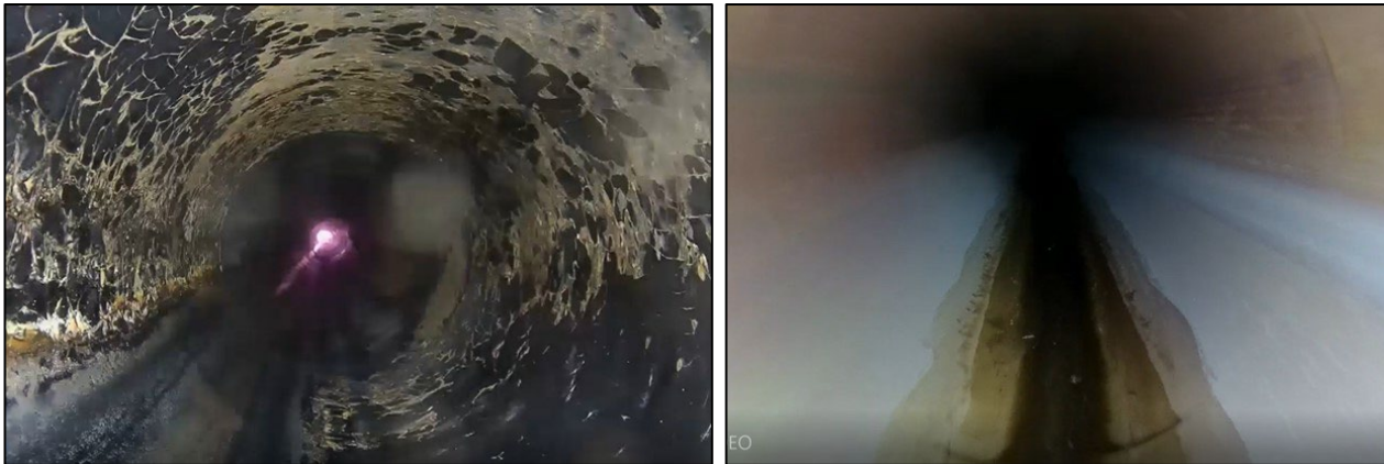
Minturn interceptor aerial crossing rehabilitation (failed interior pipe coating right, completed rehabilitation right)
