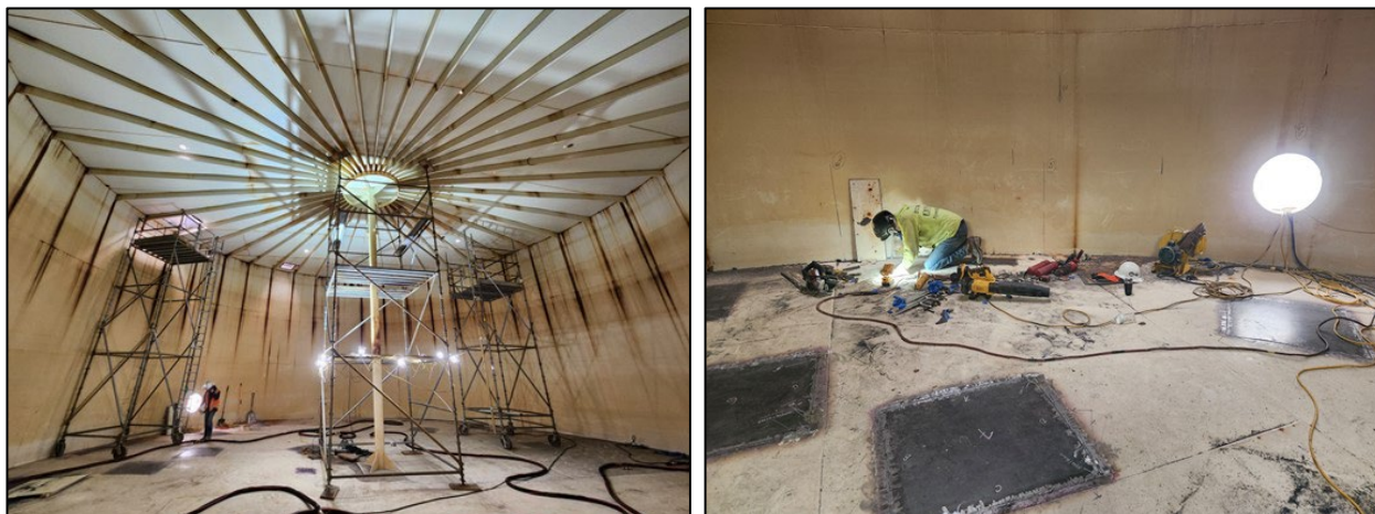
Cordillera West Tank 1 rehabilitation (temporary interior scaffolding installation left, floor repairs right)
