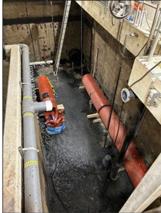
Mixed liquor pipe replacement at VWW (new pipe shown on right side of photo)
