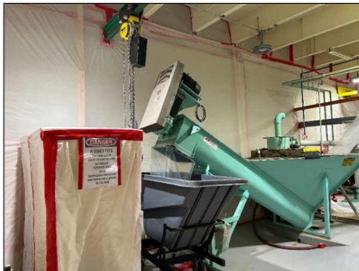
Asbestos containment barriers installed in VWW headworks
