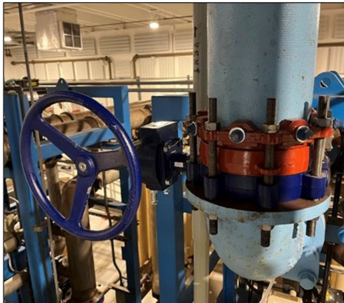
EDWF membrane system “block-and-bleed” valve installation
