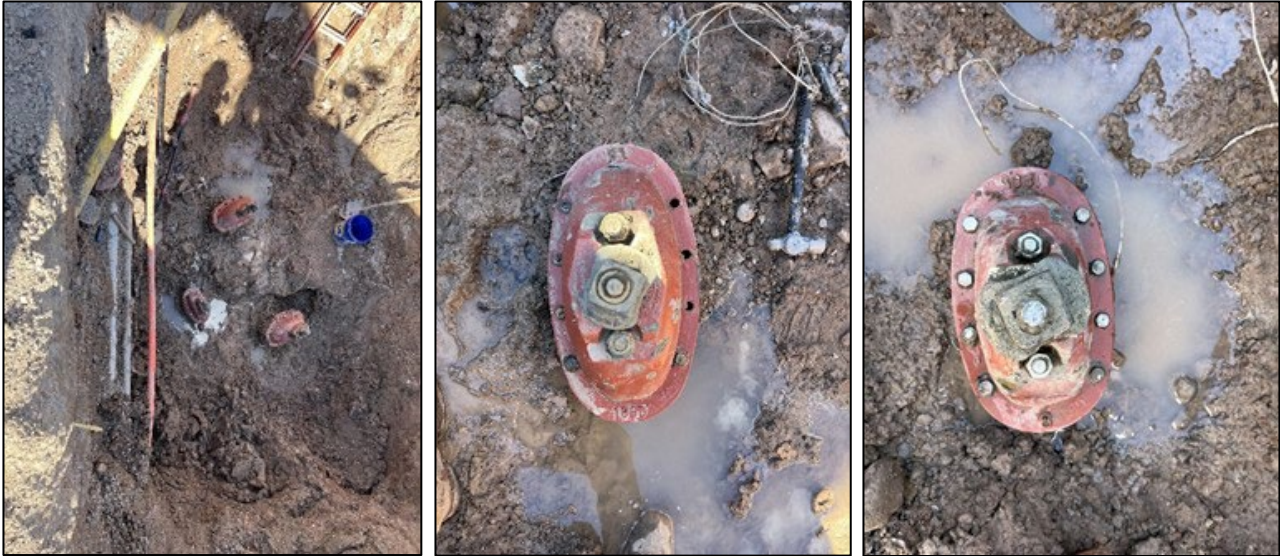
Beard Creek Trail Road water valve repair (excavation left; valve with corroded bolts middle, completed repair right)
