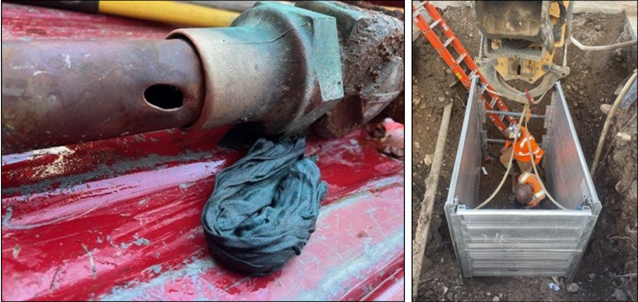
East Vail water service repair (pipe damage left; service repair in-progress right)
