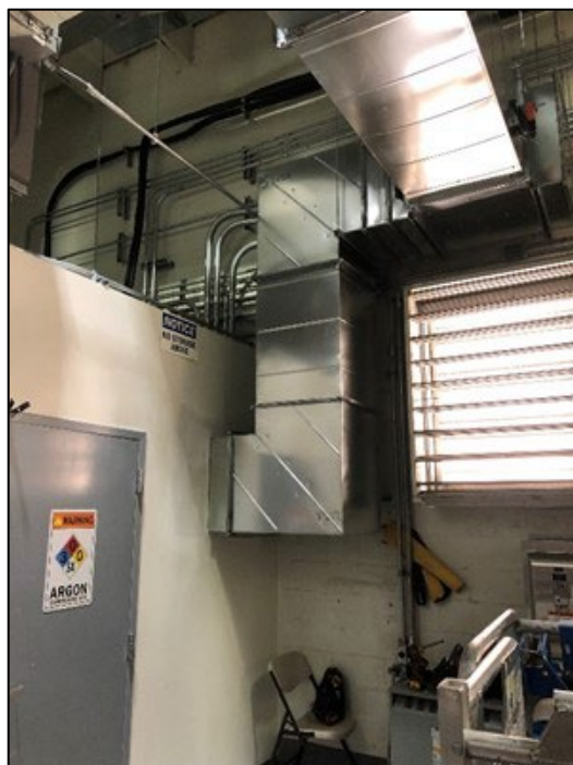
New ductwork routed from an existing HVAC unit (to temporarily cool the server room)
