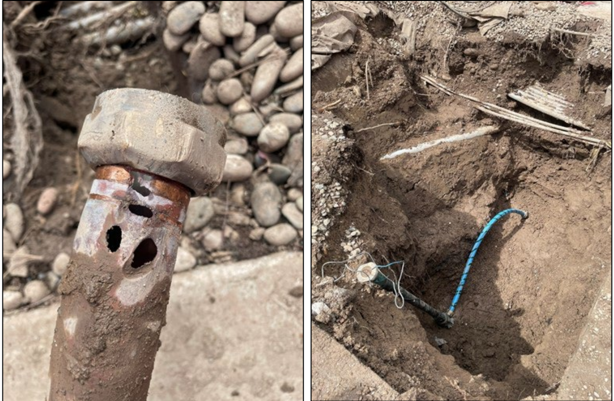
Stillwater water service repair (pipe damage left; repaired service pipe right)
