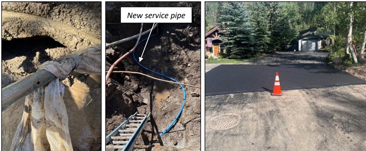
Main Gore Drive water service repair (pipe damage left; service line replacement middle, completed repair right)
