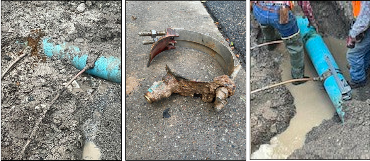
Edwards Village Drive water service repair (pipe damage left; corroded saddle middle, repair right)
