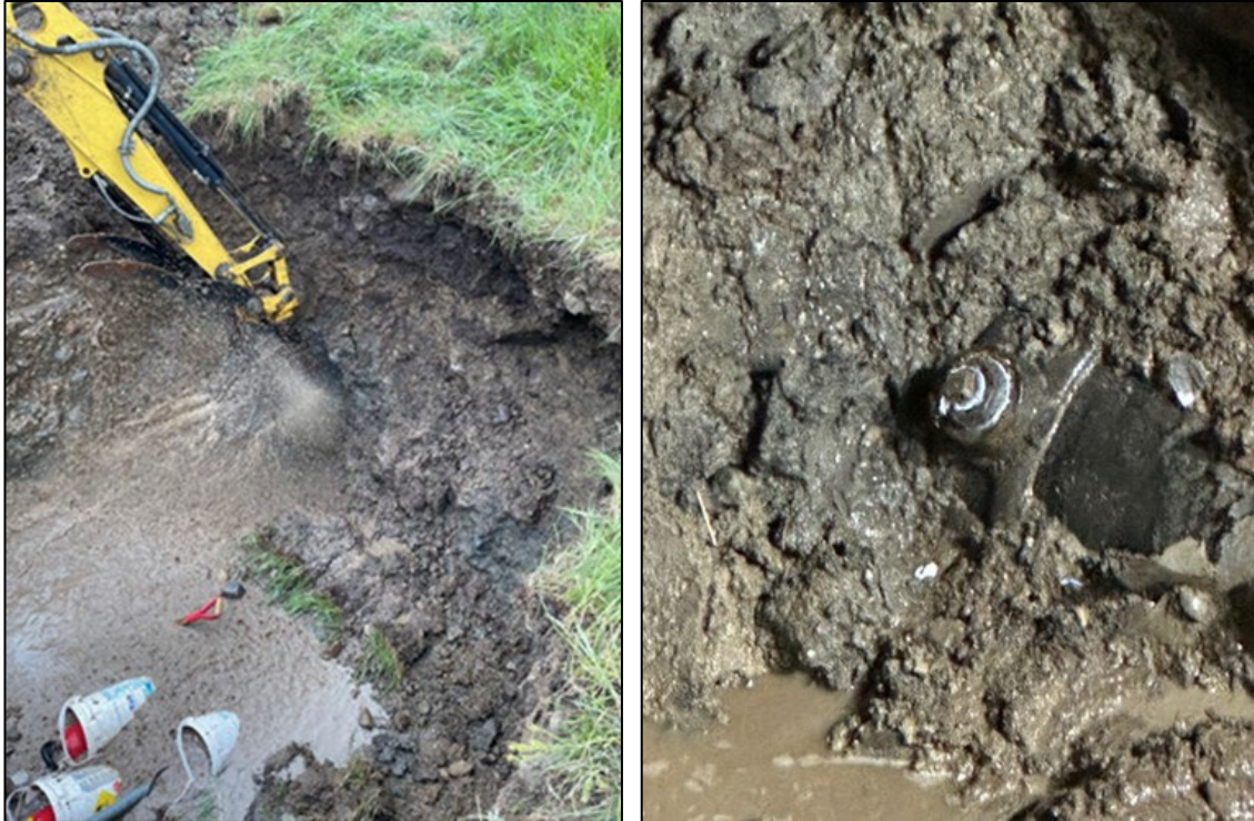
Beaver Creek Golf Course water service repair (excavation and pipe damage left; repair right)
