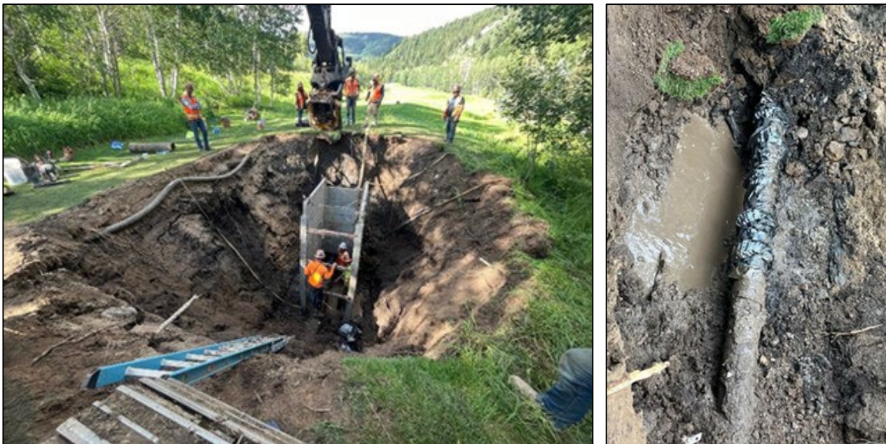
Beaver Creek Golf Course water main repair (excavation left; repaired pipe right)
