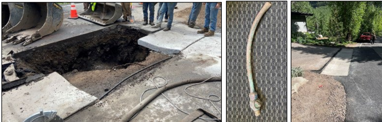
East Vail water main repair (excavation left; damaged service center, completed repair right)
