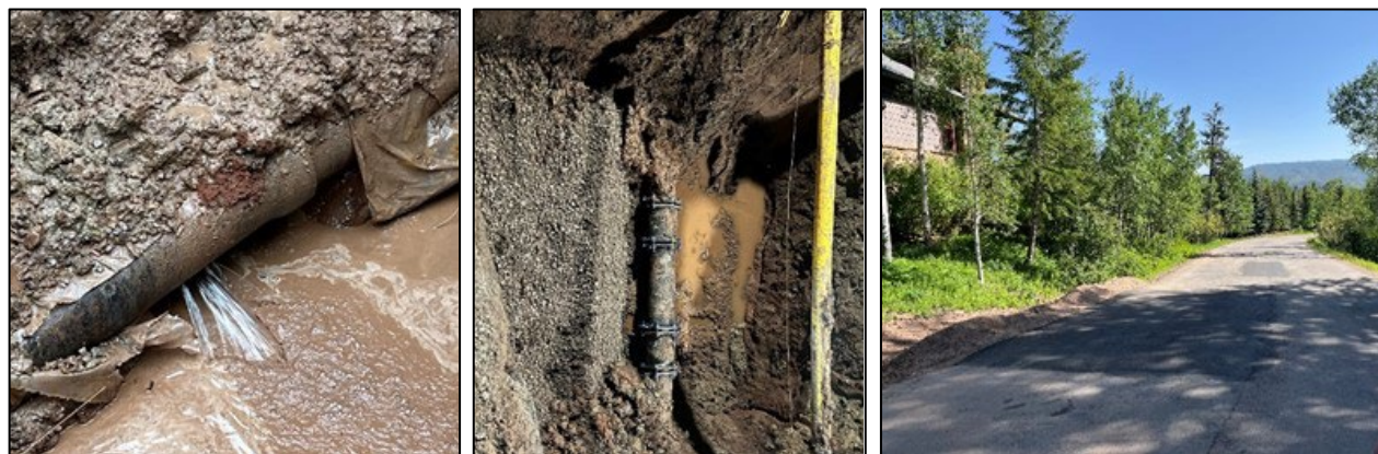
Cordillera water main repair (damaged pipe left, repaired pipe center; completed repair right)
