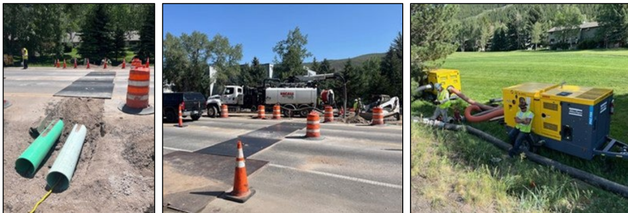
Avon sewer collection interceptor bypass pumping and cleaning project (temporary bypass pipe left, jetting equipment center, bypass pumps right)
