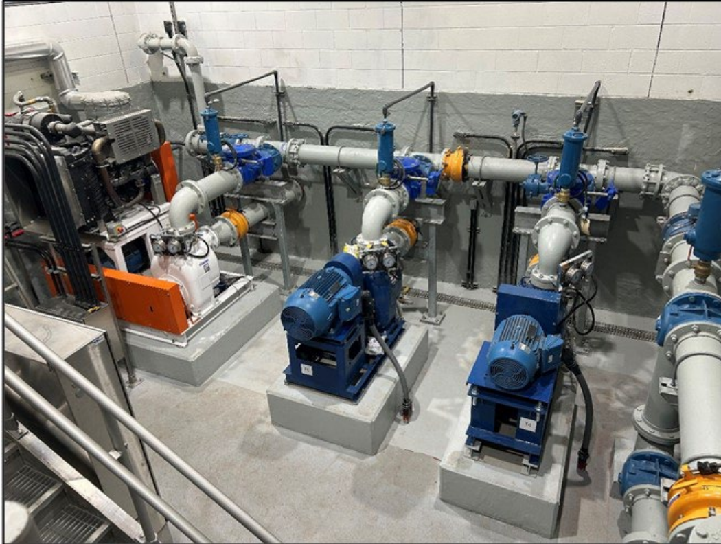
Interior view of completed lift station
